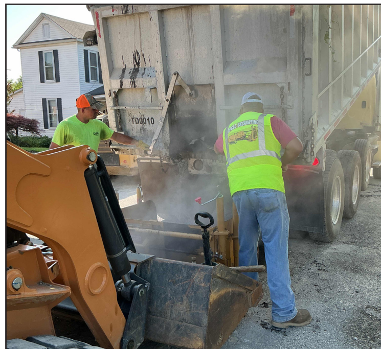
Crews work on the water line replacement in Grayson using the asphalt attachment for the skid steer. (submitted photo)
