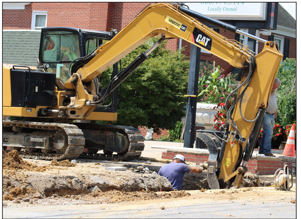
Crews work on the water line replacement project earlier this summer. (File photo by Jeremy D. Wells, Carter County Times)
