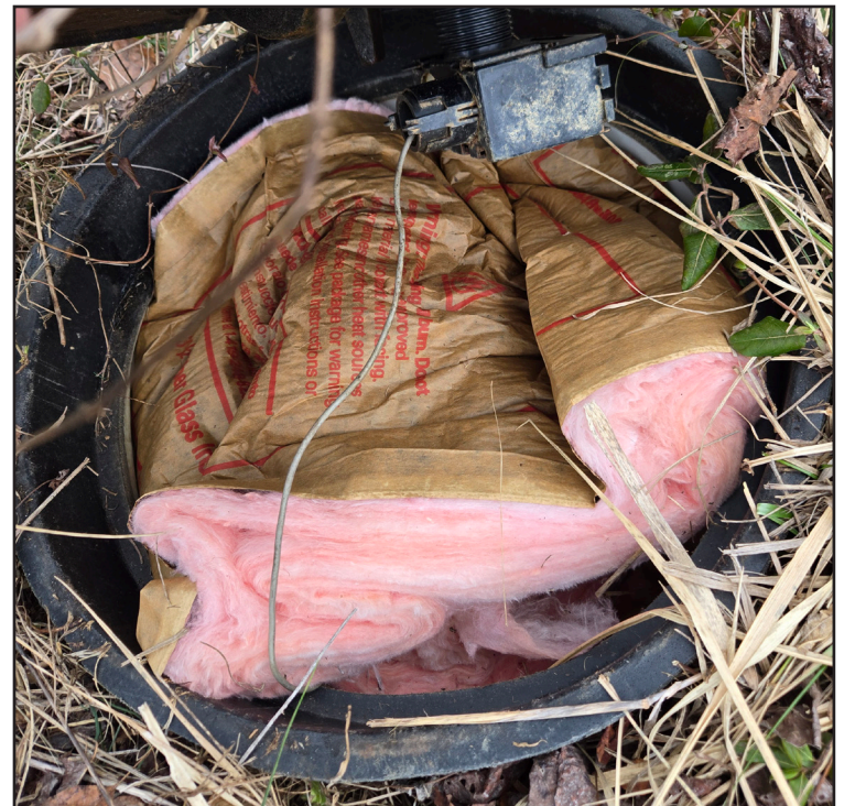
Insulation covers a water meter to prevent freezing. (Photo by Jeremy D. Wells, Carter County Times)
