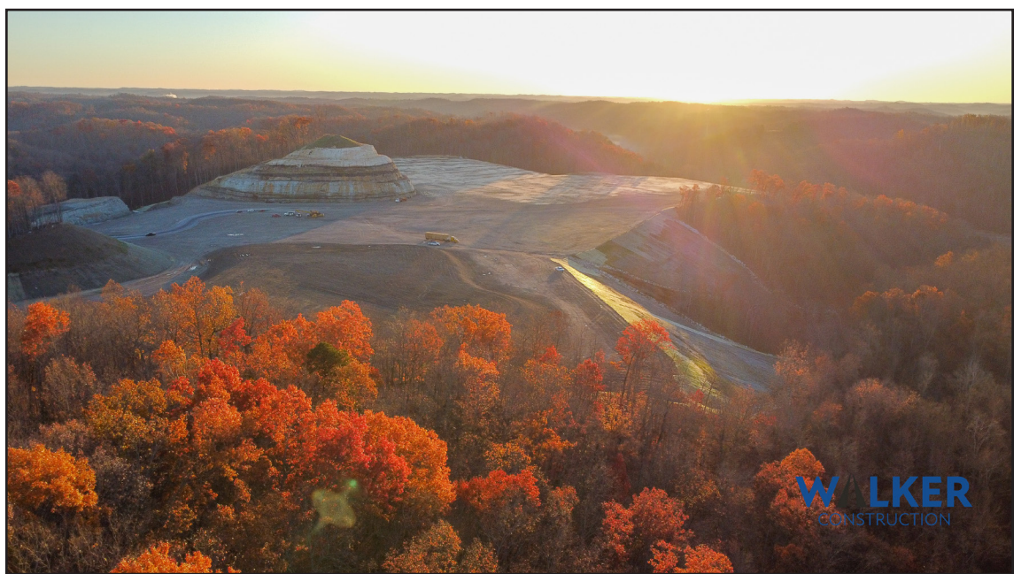
While site preparation for the new high school has proven to be more expensive than anticipated, a new phased construction plan could keep date-dependent funds from being clawed back. (submitted photo)
