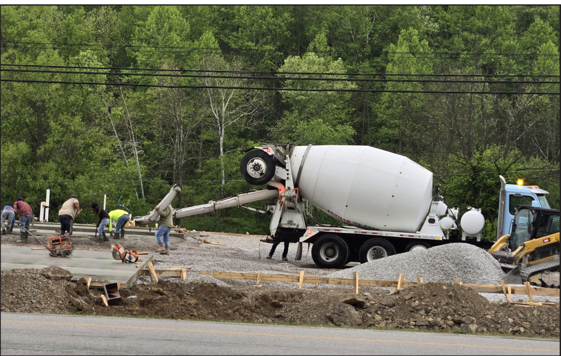
The proposed data center is expected to create several construction jobs during the buildout phase. (File photo by Jeremy D. Wells, Carter County Times )
