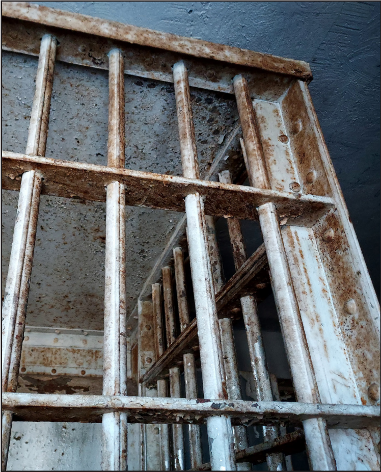
Conditions inside the old jail are beyond repair and the building has become a safety hazard, according to the fiscal court. (File photo by Jeremy D. Wells, Carter County Times )
